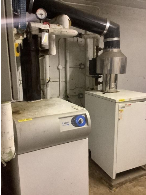
Existing Gas Fired Boilers
