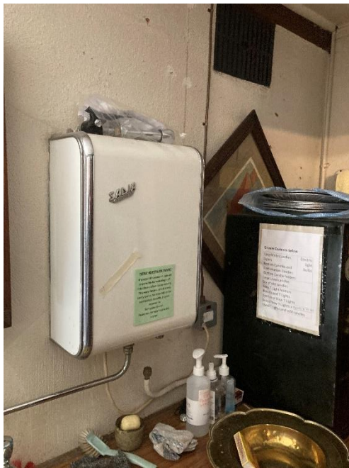
Existing Electric Water Heater in Vestry
