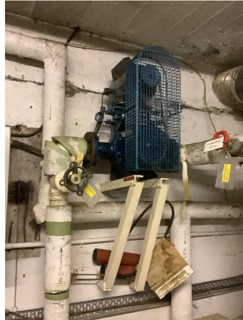
Existing Belt Driven Pump
