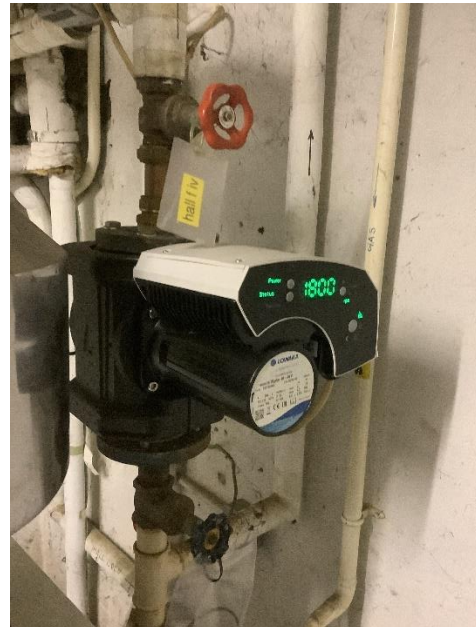
Existing Inverter Driven Pump
