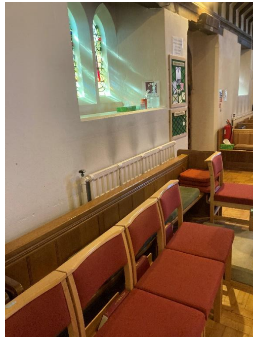
Existing Single Panel Radiator in Church
