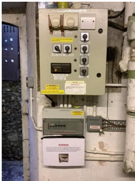
Existing Control Panel
