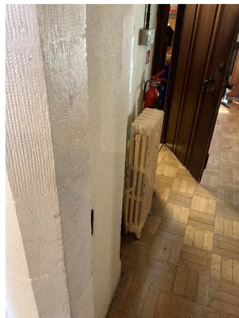
Existing Column Radiator in Church
