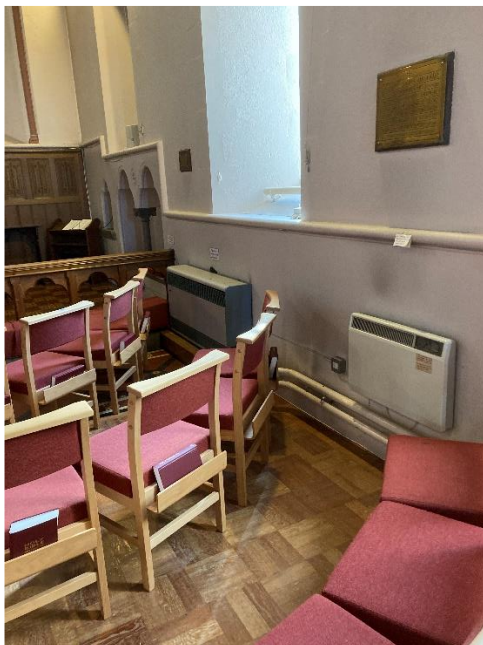
Existing Electric Heater and Fan Convactor
